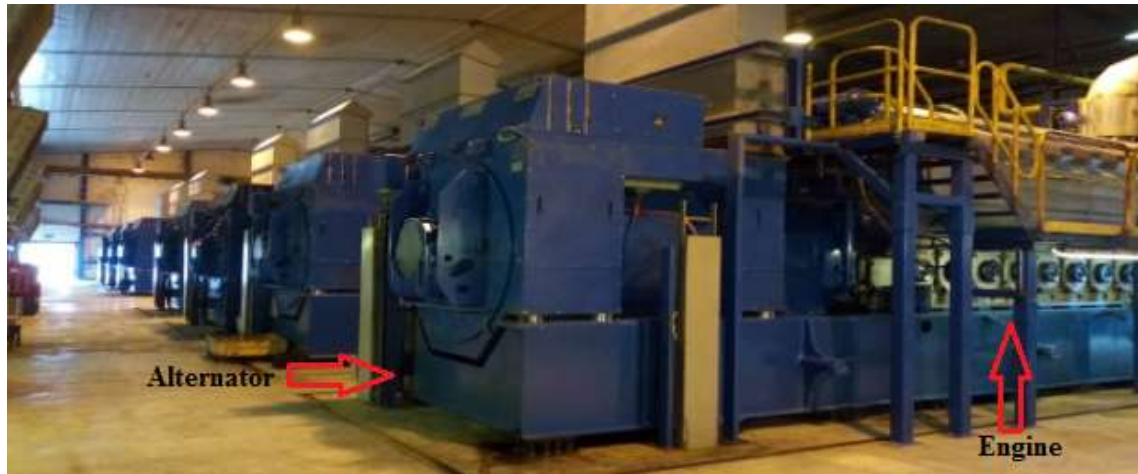
Figure: 2 The machine room
